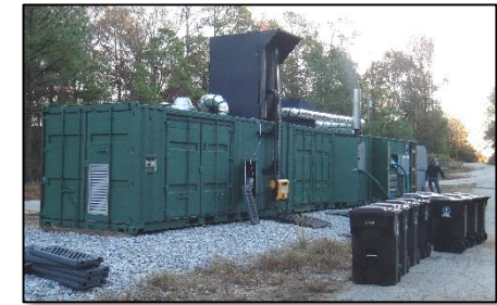
MSW Power BWEC
