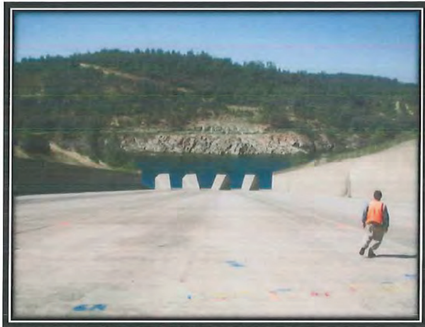
21. The lower flood control outlet chute is shown. Not the markings for the upcoming chute repairs. 6/25/10 Inspection Report
