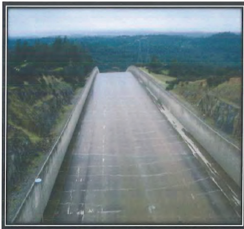
12. The concrete along the spillway chute has been repaired. The repaired herringbone crack pattern is said to reflect the underlying drain system.
