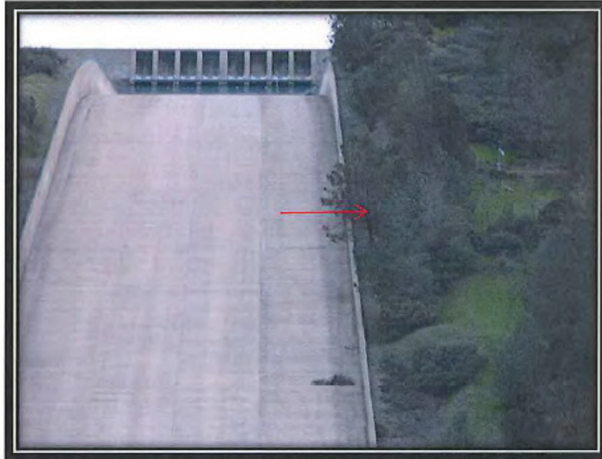
9. This view looking upstream along the FCO discharge chute shows one tree (arrow) that needs to be removed following a significant effort to remove brush along the outside of the wall.
