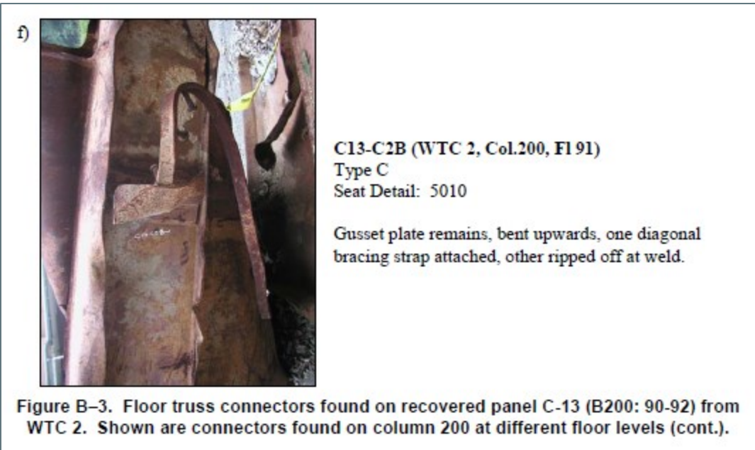
Figure 24: A perimeter column to floor truss connection from floor 91 of the South Tower ("Zone 1") indicates upward acting forces that bent the seat upward as the destruction moved upward.
