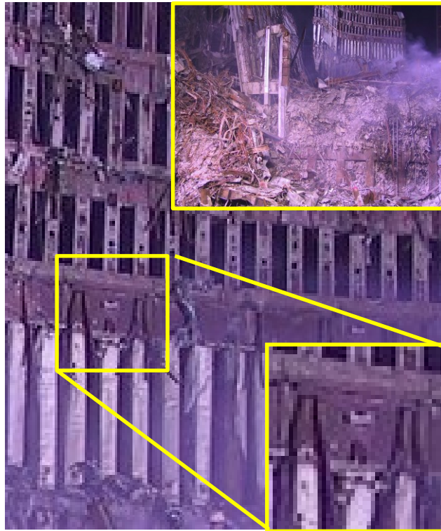
Figure 46: Inner perimeter columns in "Zone 3" of the North Tower showing hanging floor truss top chords.
