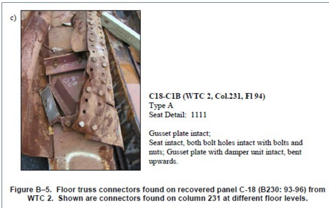
Figure 23: A perimeter column floor truss connection from floor 94 of the North Tower ("Zone 1") indicates upward acting forces that bend the seat upward as the destruction moves upward.
