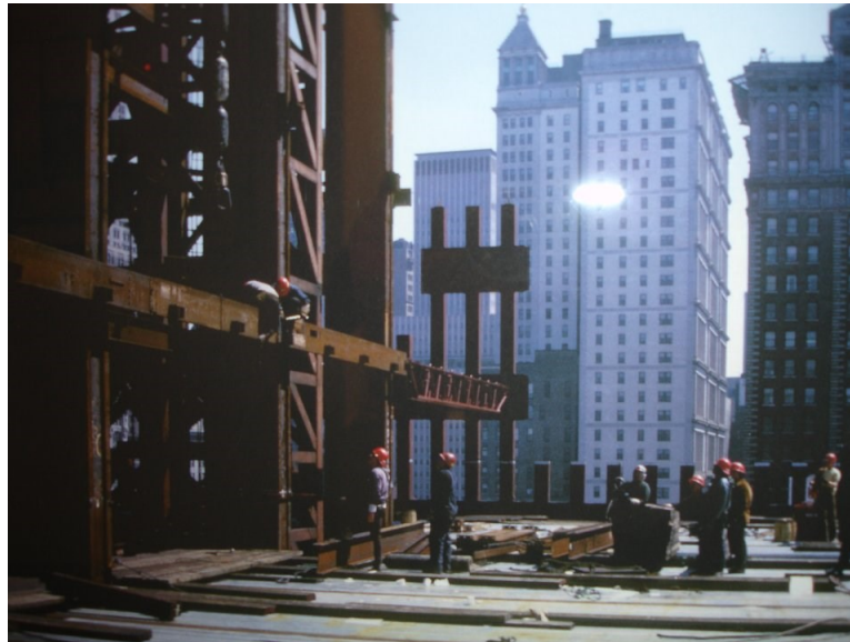
Figure 20: Photo showing a channel with floor truss seats. A floor truss connecting the channel to a perimeter column is shown at the far end of the construction zone.
