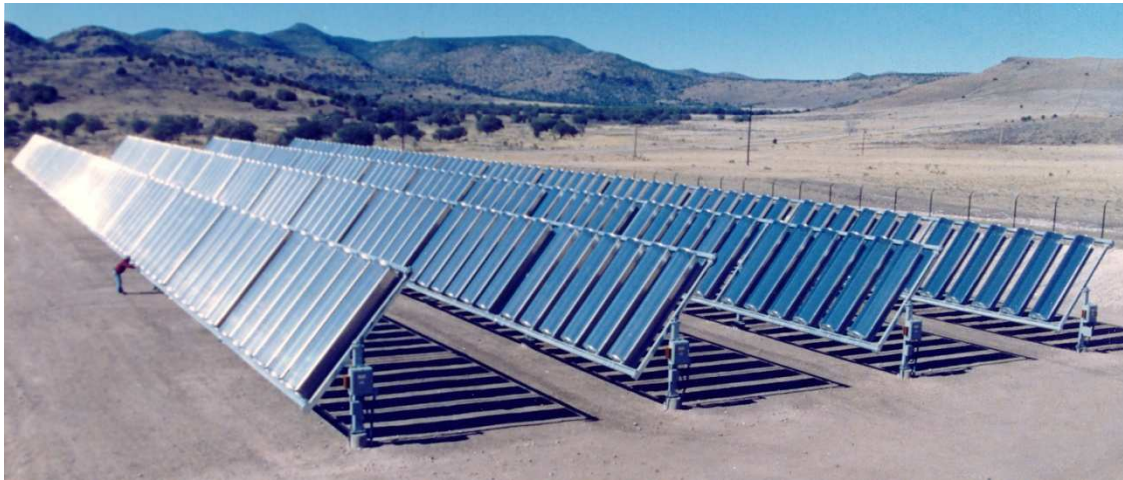
Four SolarRow™ Trackers for Previous Generation of Entech CPV Modules
