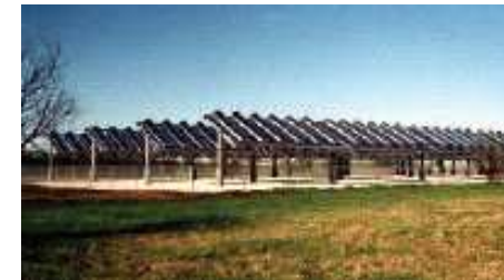
TU Electric (Texas Utilities Company) 100 kW CPV System
