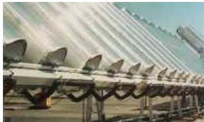
Sandia National Labs 10 kW and 22 kW CPV & CPVT Systems
