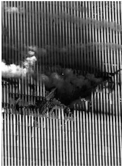
Fig. 1. A “clean” cut driven by the wings of a Boeing 767 into the facade of the North Tower.
