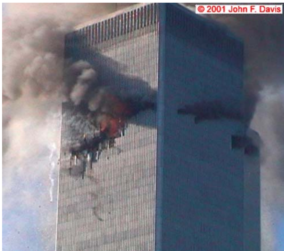
Figure 2–2. Aircraft entry hole on the north side of WTC 1, photographed 30 s after impact.
